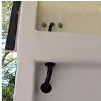
All wires that run through chassis are grommited
